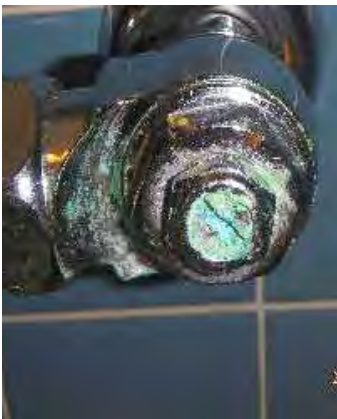
P.12 – Corroded flush valve
