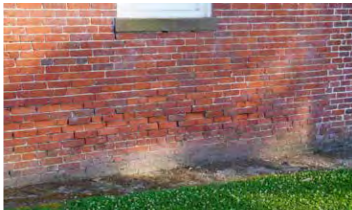
Brick masonry damage at north wall of historic courthouse
