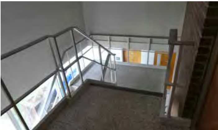
Code-compliant guardrails not provided at stairwells
