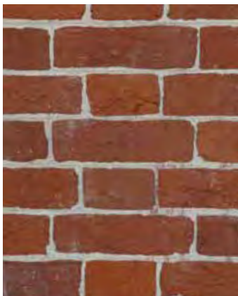
Damaged historic courthouse brick
