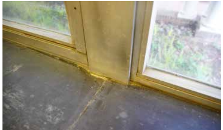
Typical interior moisture damage at 1960s ribbon windows
