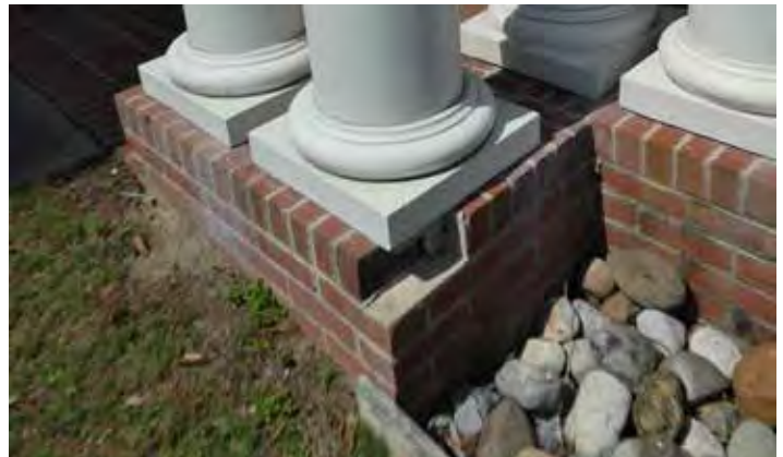
Ground gutter and missing knee wall brick at breezeway
