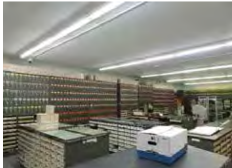
E.12 – Records Room: T8 linear fluorescent light fixtures
