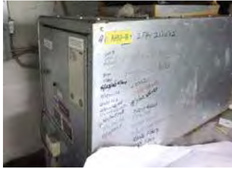
M.5 – Air handling unit AHU-9
