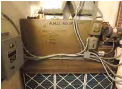
M.9 – Air handling unit AHU-8
