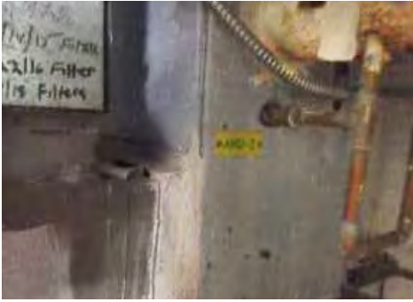
M.4 – Air handling unit AHU-2
