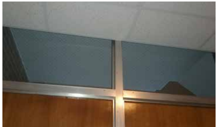
View from lobby of retrofitted drop ceiling and unrated aluminum storefront frame/glazing/wood veneer panels at stairwell
