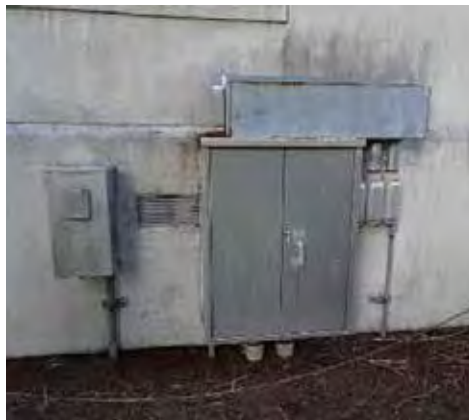
E.2 – CT cabinet/meter for 208Y/120V, 3Ø service
