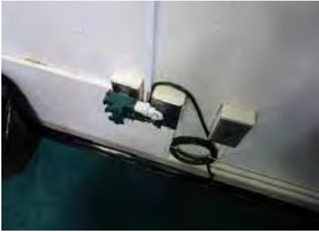
E.20 – Two 3-way outlet wall plugs
