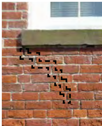
Diagonal masonry and mortar cracking at window 8
