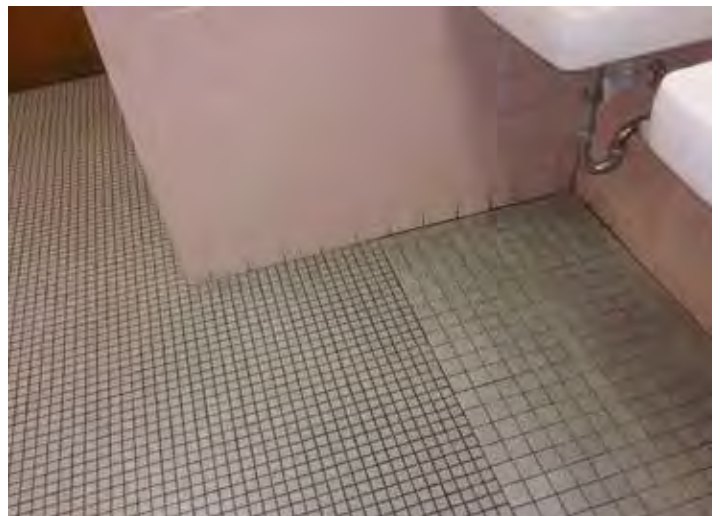
Wall and floor tile in first-floor women's restroom (similar in men's restroom across hall); tile type transition indicates possible repair made for previous moisture damage (correlates with moisture issues reported at this wall)
