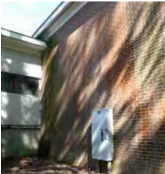
Brick discoloration at north wall of one-story 1960s addition
