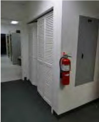
Malfunctioning residential-grade accordion-fold closet door
