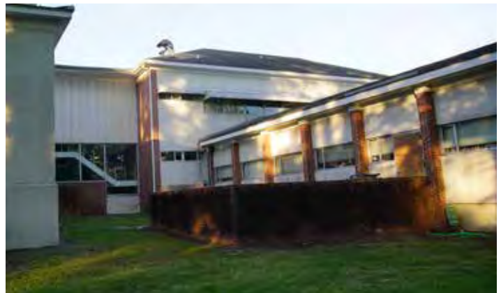
Stained and damp masonry site wall with organic growth; rusted exterior door; sunshades at west-facing windows
