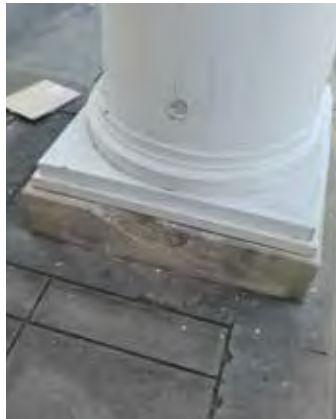
Cosmetic damage to stone column base; detail of column stave splitting
