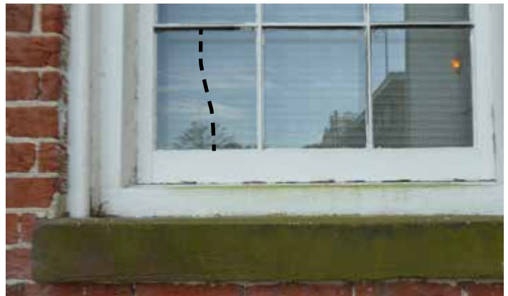
Broken pane at window 5; organic growth on stone sills typical; deteriorated bottom rail typical
