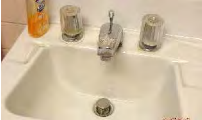
P.9 – Corroded lavatory / faucet
