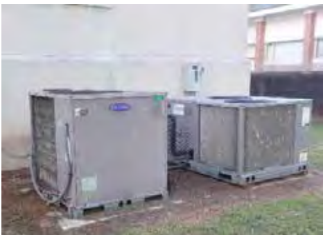
M.1 – Carrier DX outdoor cooling units
