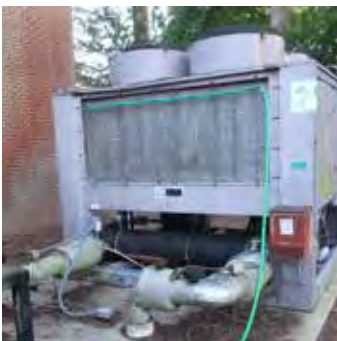
M.12 – Air-cooled reciprocating chiller
