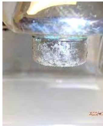
P.13 – Corroded lavatory faucet aerator
