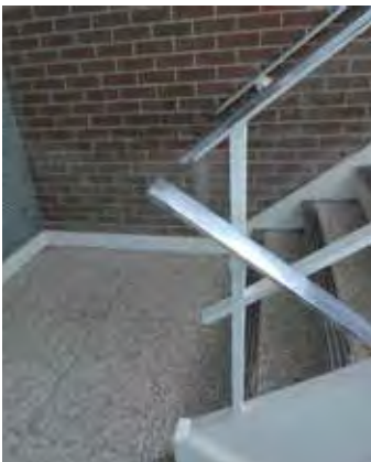
Discontinuous handrail, no guardrail in south exit stair
