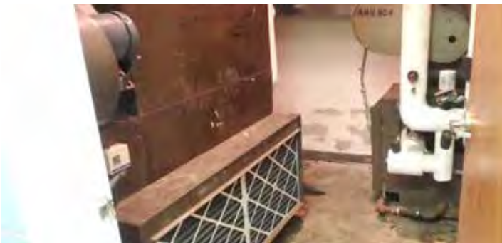
M.7 – Air-handling units AHU-3 and AHU-4
