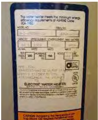
P.5 – Water heater nameplate
