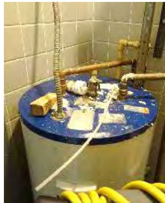
P.2 – Corroded pipe
