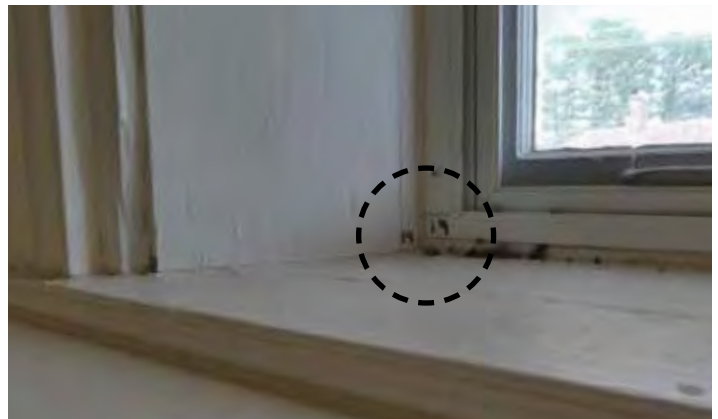
Typical numerical label at window jamb and interior storm window with screen; splitting of wood sill and minor wood trim damage evident
