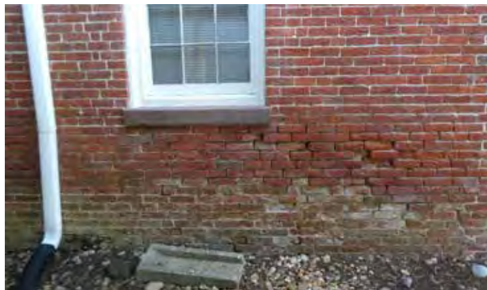
Brick masonry damage at south wall of historic courthouse; splash block is improperly located (and likely inadequate) to divert rainwater
