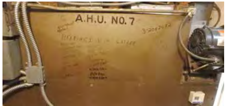
M.8 – Air handling unit AHU-7
