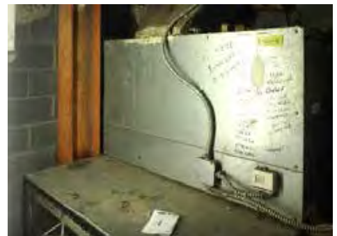
M.3 – Air handling unit AHU-3
