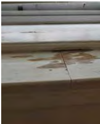
Moisture damage at interior sill of window 14
