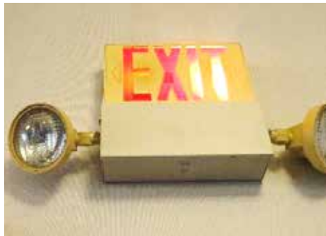
E.15 – Incandescent exit sign with emergency lamps
