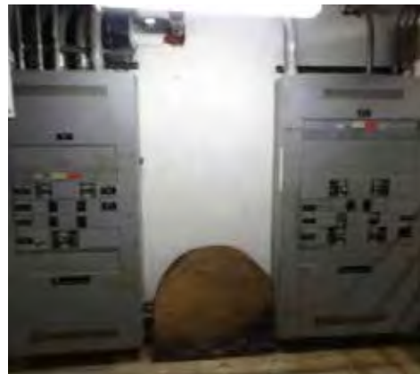
E.3 – Basement: 1200A Main Distribution Panel 1 (MDP1) & 400A Main Distribution Panel 2 (MDP2)
