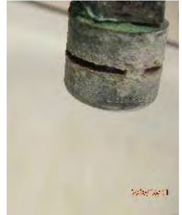
P.11 – Corroded lavatory faucet aerator
