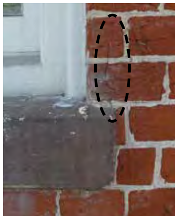
Vertical masonry cracking at window 1
