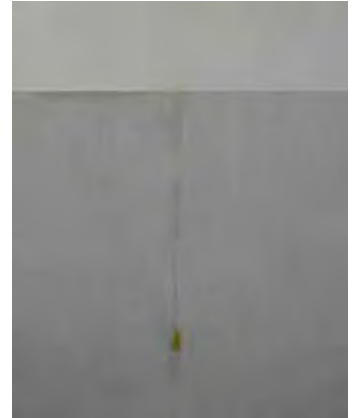
Damaged vinyl wallcovering wainscoting in first-floor corridor
