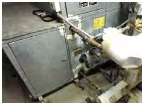
M.2 – Air handling unit AHU-1
