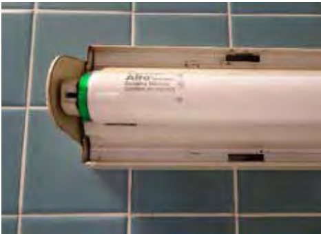
E.11 – Bathroom: T12 linear fluorescent
