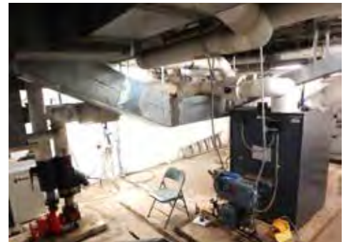
M.11 – Fuel oil boiler & HW pump in basement
