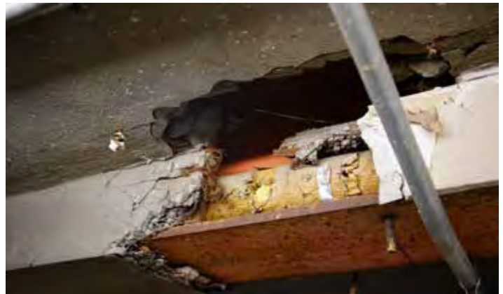
Fireprotection deterioration at overhead beam in basement
