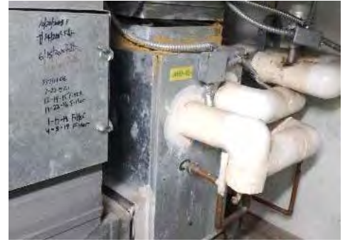
M.6 – Air handling unit AHU-10
