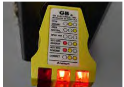
E.19 – Properly grounded receptacle
