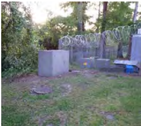
E.1 – 3000 KVA pad-mounted transformer
