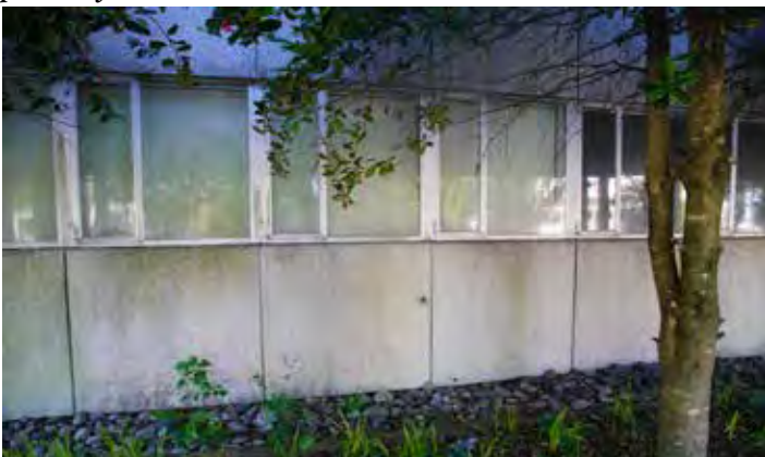
View of first-floor 1960s ribbon windows from east; windows are shaded by vegetation; stone aggregate ground gutter collects roof drainage
