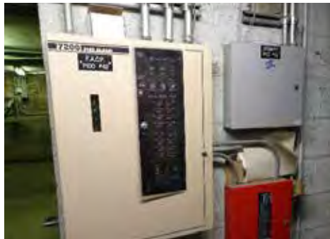
E.28 – Fire alarm control panel, security panel, and digital alarm communicator transmitter
