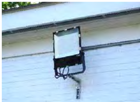
E.18 – Exterior: Wall-mounted LED
