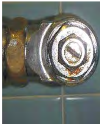
P.14 – Rusted flush valve
