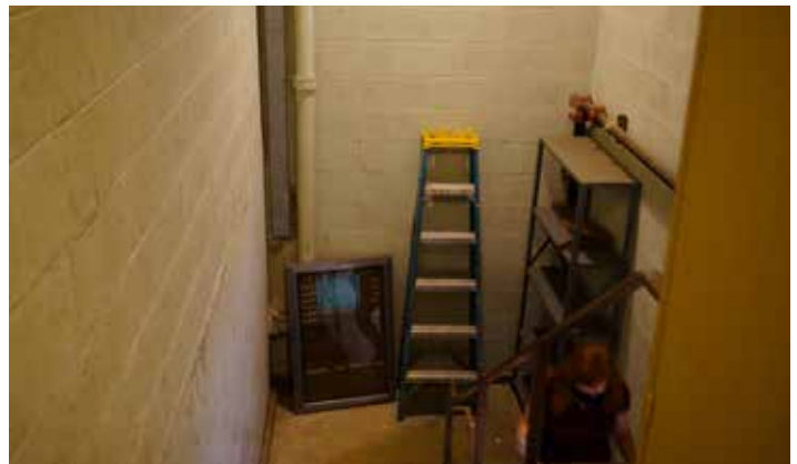
Items stored in stair to basement are an egress hazard
