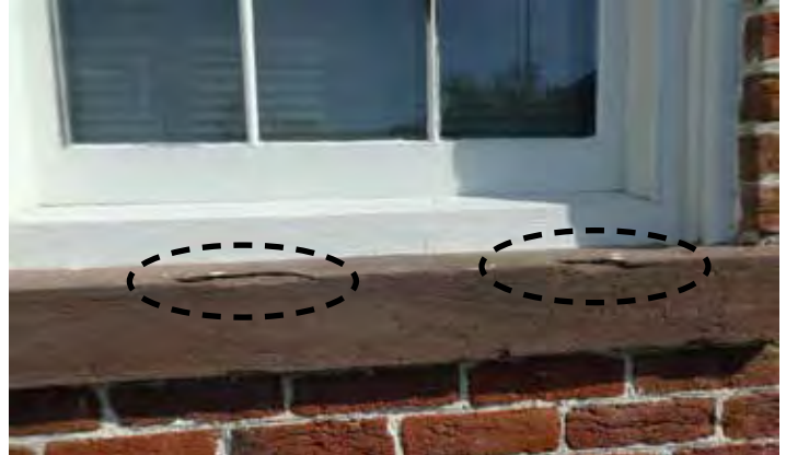
Sill damage at window 7
